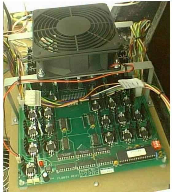
Fan Assisted Cooling
